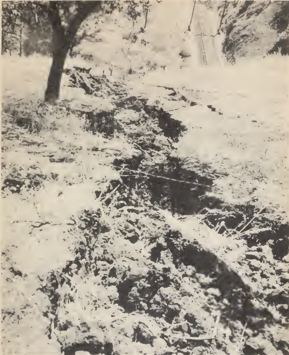
FIGURE 31. Crack in earth above Tunnel 4, Southern Pacific Railroad. Photo courtesy Southern Pacific Railroad.
